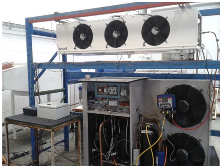
Figure 3 - Evaporator and Condensing Unit
